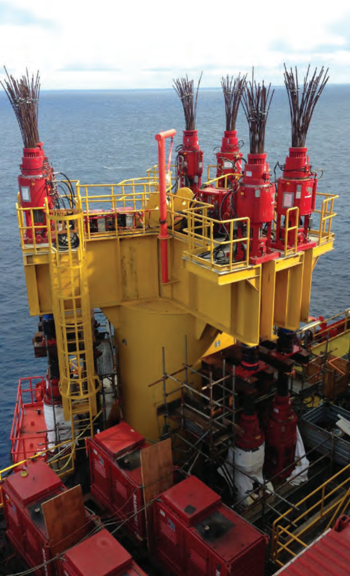
Close-up: Mammoet strand jacks and power packs installed on the platform legs
