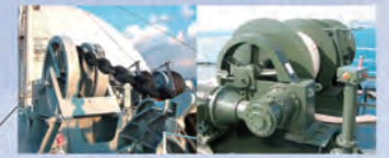
ELECTRO-HYDRAULIC DECK MACHINERY (WINDLASS/MOORING WINCH)
