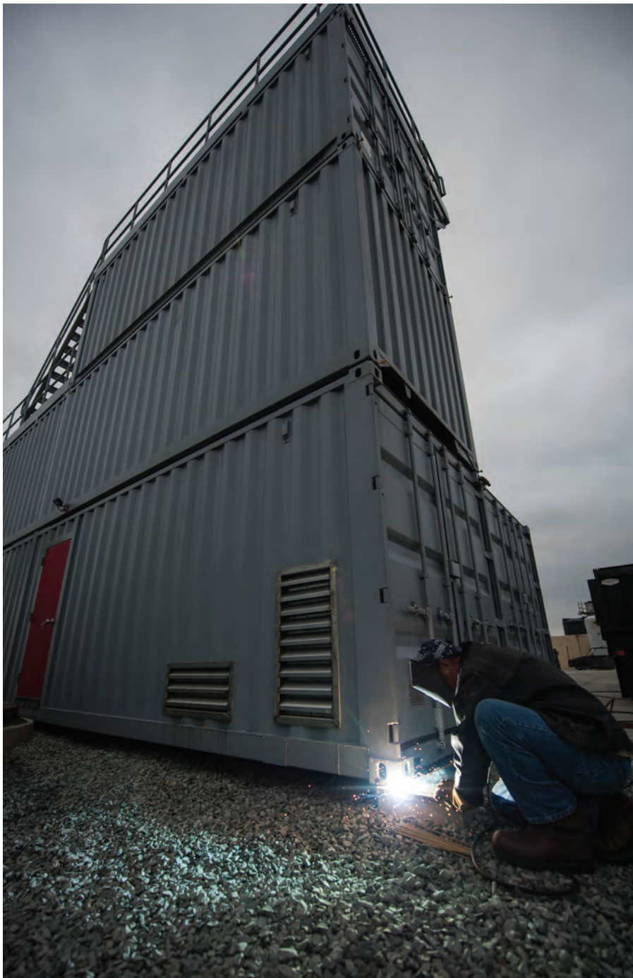
Nick Lugue Jr., a welder with Naval Facilities Engineering Command Southwest, welds a new firefighting trainer into place at Naval Air Station North Island. The trainer is the first of four new trainers the Navy is building that will simulate potential fire hazards aboard submarines. (U.S. Navy photo by Mass Communication Specialist 3rd Class Todd C. Behrman)
