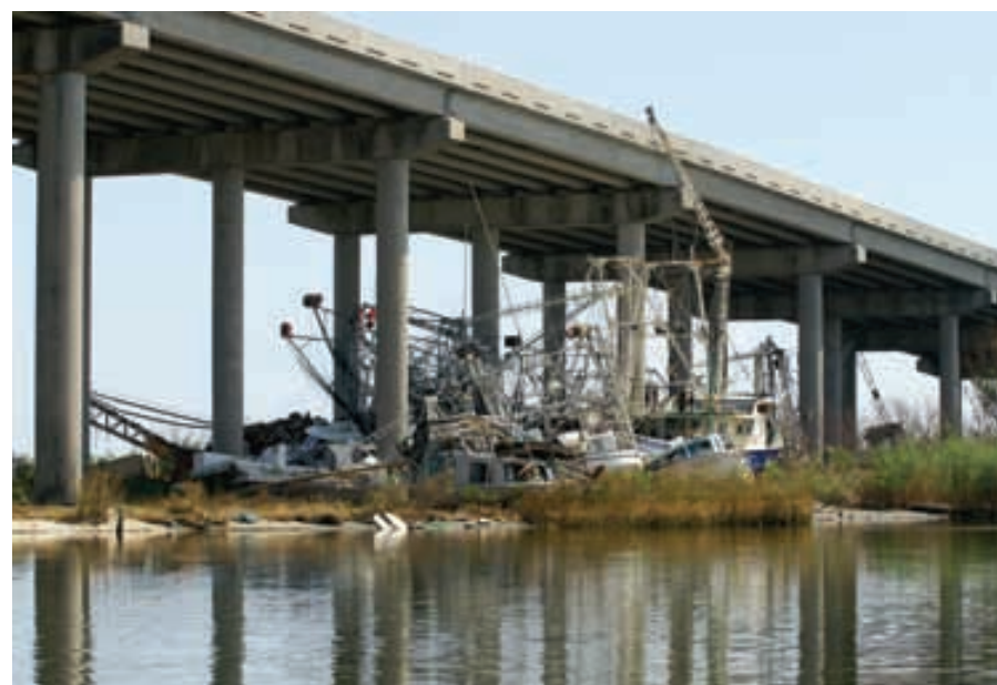
The overpass near Empire, with the broken hulls and tangled outriggers of shrimpers marking where the surge met the highway structure, shoving then dropping whatever was on its course. (Photo: Don Sutherland)
