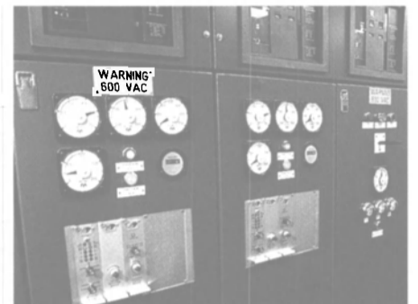
Close-up shot of SCR cabinet.
