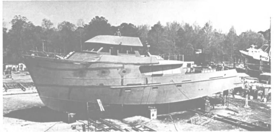
Despite its size, the luxurious Alpha Centauri draws only 6 feet. Shown under construction at Freeport Shipbuilding in Florida, the yacht will have a 10-foot by 27-foot "sports platform" extending from the stern that can accommodate divers, fishermen and equipment.
