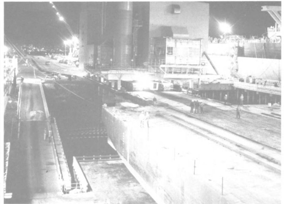
The modules were moved by crawlers over a specially prepared roadway to a loading dock leading onto the barges as each was positioned on Dry Dock 4.
