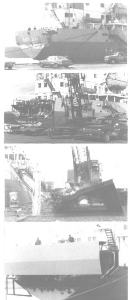
Photos, top to bottom: The M/V Saint Jean showing damage sustained to her stern transom plating; The Saint Jean after her damaged plating has been removed; Enterprise Marine employees shown performing work on the vessel's new steel; The Saint Jean's new stern transom plating is lowered into place.
