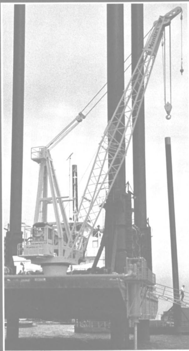
ABOVE: Mounted onboard the jack-up barge M/V Ben Tolbert, this Manitex ML-4800 is rigged with an 80' boom to perform offshore repair work throughout the Gulf of Mexico.
