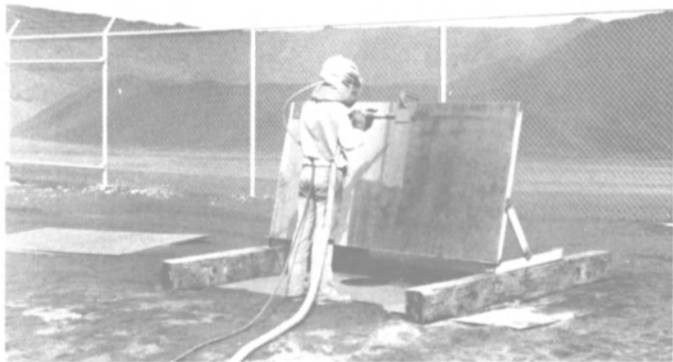
COPPER BLAST (in use here) has very little dust, is low in free silica, cuts 30-50% better than lower-quality slag abrasives and up to four times better than many silica sands.
