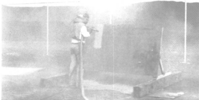
Dust (shown here from silica sand) means lower cutting efficiency and visibility and increased health hazards and clean-up costs
