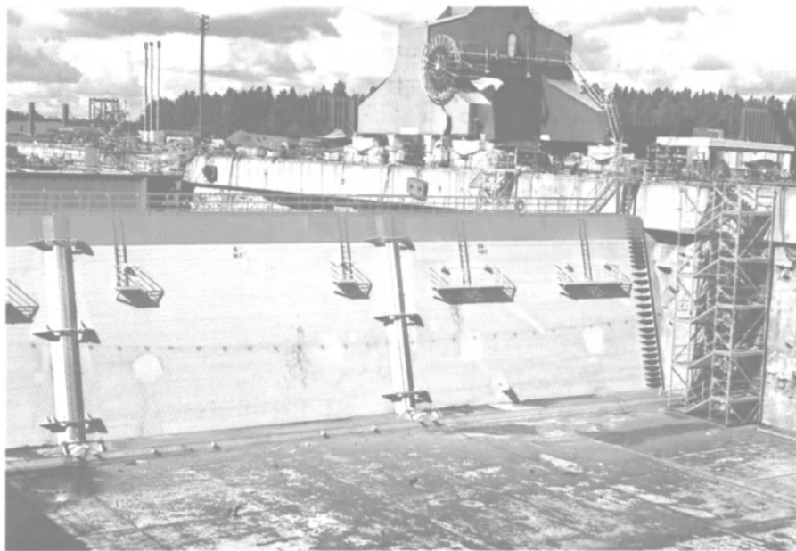
New intermediate dock gate at Valmet's Helsinki yard. This gate has turned this large drydock into both a newbuilding and repair dock, with the Finnish yard being capable of repairing vessels of up to 60,000 dwt in this 'new' facility. Photo—M. Hood.
