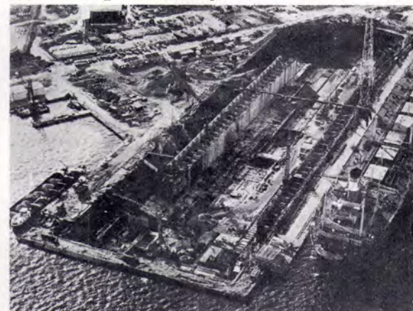
The graving dock presently under construction at Mercantile Engineering & Graving Docks Co., Antwerp. It is expected the dock will be operational in September.
