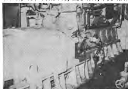
DIESEL GENERATOR SET
