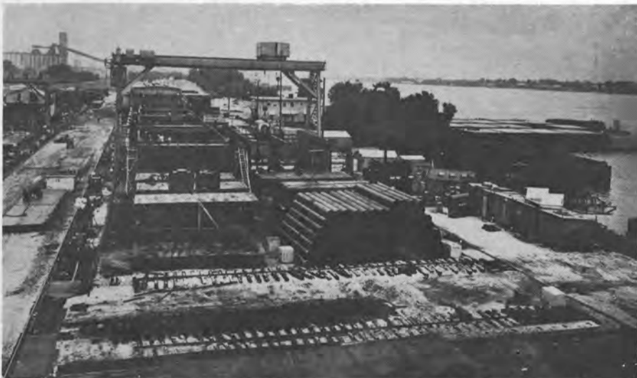
LASH lighter assembly lines at the Westwego plant of Avondale Shipyards are turning out two lighters daily. Fabricated lighter sections are assembled, sandblasted, and painted on their way to the launching ramp. Avondale is presently working under contracts to provide a total of 821 lighters for two steamship companies.
