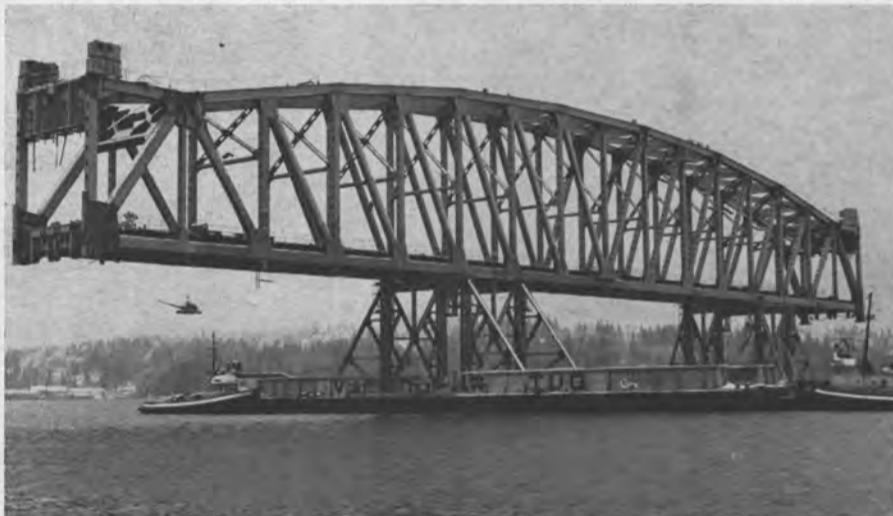
2. The lift span, weighing 2,400 tons and 503 feet long, is the largest of its type in Canada and the fifth largest in the world. It is believed to be the first time that a lift span of such size has been floated into place by this method. The sections were assembled on ways by Canron Limited, about 4½ miles from bridge site.
