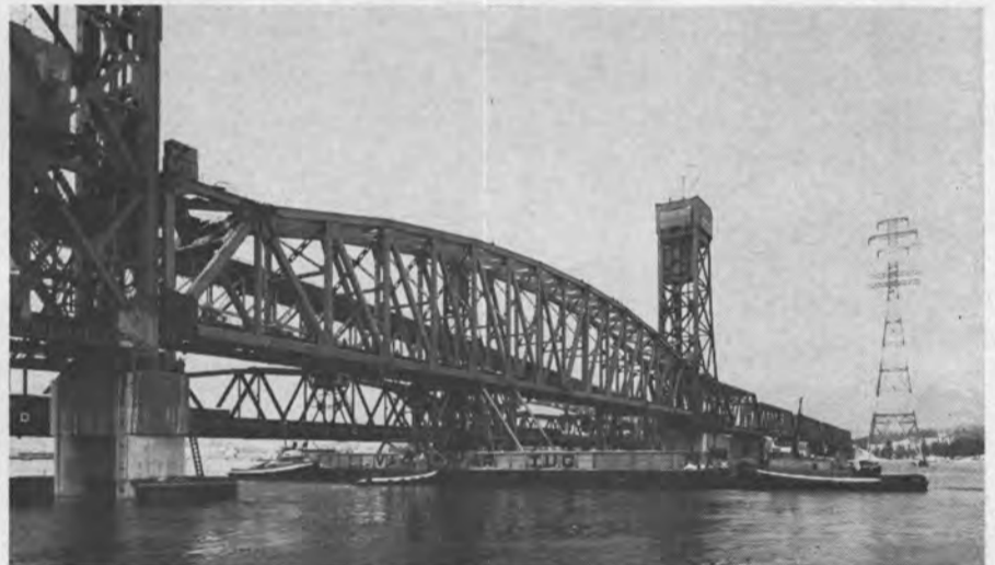
4. As the tide fell, ballast was pumped into the barges and the bridge section lowered onto the supports. The new bridge is scheduled to commence carrying railway trains this spring. Tugs, La Belle, Le Prince, La Fille, and La Lutte, were used for this operation together with the 260-foot VT 152 and 180-foot VT 52 barges.
