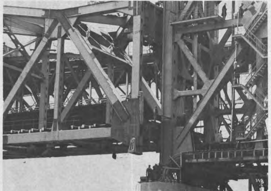
3. At the waiting pier supports, the span was gently eased into alignment with the matching structure at high tide. All of Vancouver Tug's skill and experience were needed to float the massive structure into the gap between the north and south tower spans, with only 2 or 3 inches of clearance at either end.
