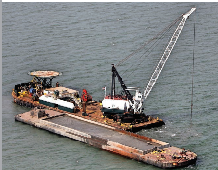
Dutra's Derrick Barge Paula Lee performs dredging work for the Port of Oakland 42 ft. deepening project.
