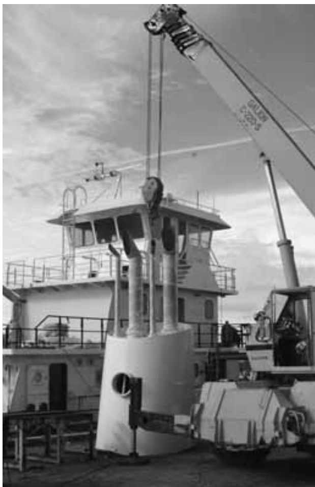
Preparing to install the stack on the towboat Rockfish. (Photo credit: Alan Haig-Brown)
