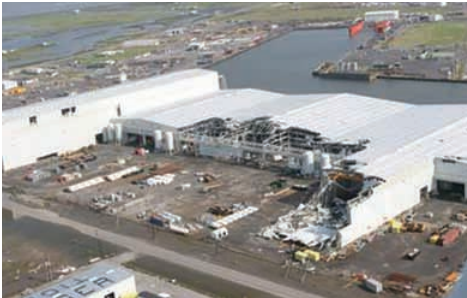
A portion of the C-Port building #2 used primarily by Edison Chouest Offshore. A portion of the building has been destroyed. (Photo Credit: Sun Herald, Biloxi)
